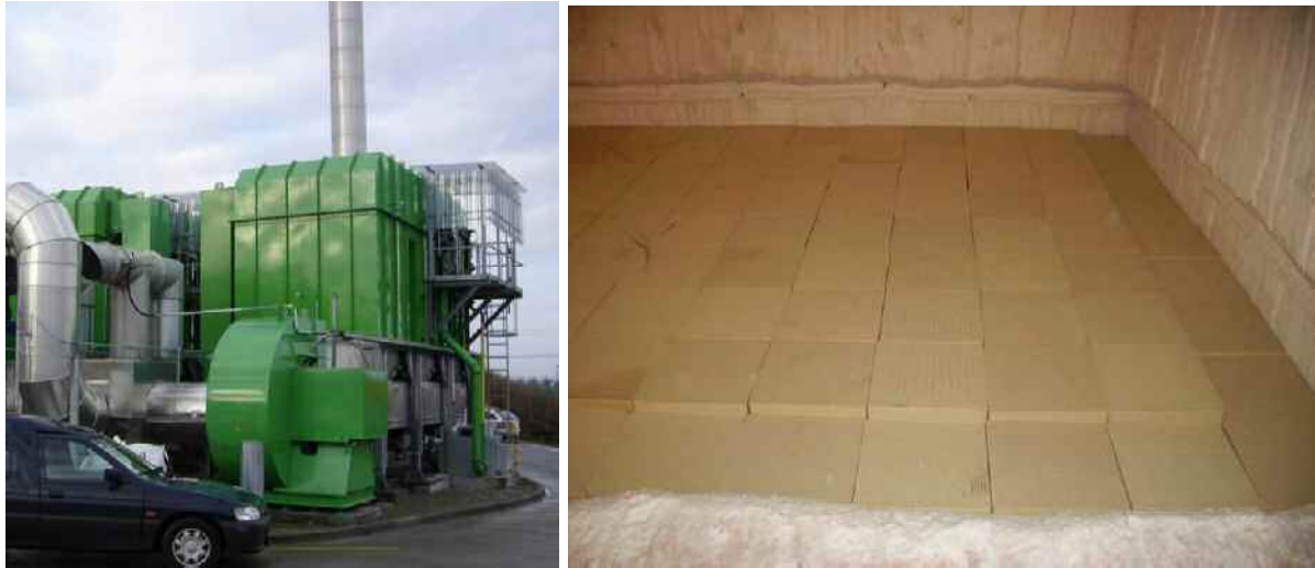
Figure 9 RTO in Stralsund and additional layer of honeycombs
