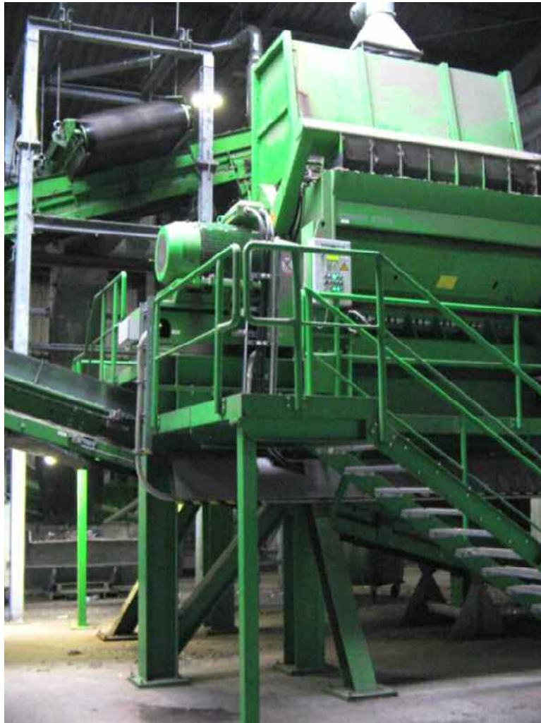
Figure 6 New post-shredder with additional magnetic separator in Stralsund
